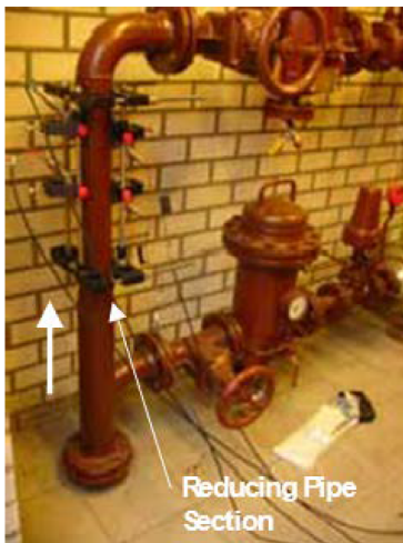
C-RL transducers installed on a 3 in (80 mm) pipe in a reducing station
