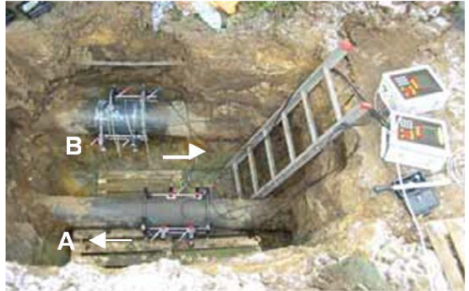
C-RL-304 (A) and 306 (B) transducers installed on pipe leading to and from the reducing station
