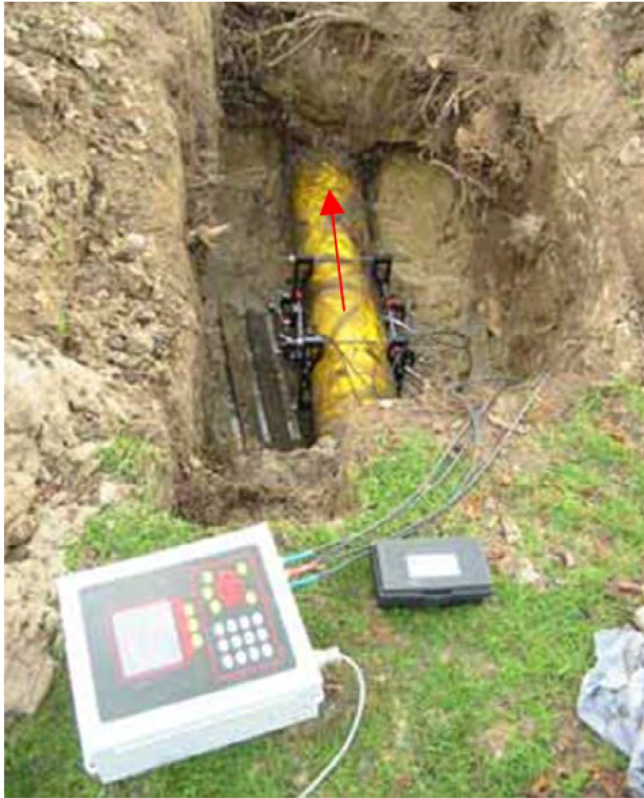
C-RL-304 Transducers installed on a 12 in. (300 mm) PVC pipe downstream of reducing station
