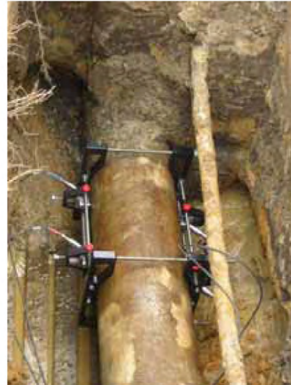
C-RL-304 transducers installed on a 12 in (300 mm) asbestos cement pipe downstream of reducing station
